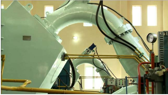
The plant and customer sites
